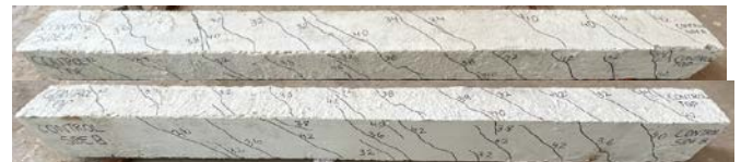
Fig 10. Continuous spiral cracks of control beam
