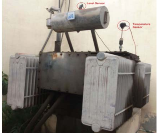
Figure 4: 400KVA DISTRIBUTION TRANSFORMER
