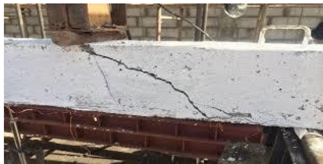
Fig 7 Failure of Retrofitted beam
