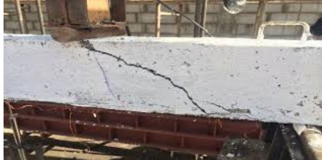
Fig 6 Failure of Retrofitted beam
