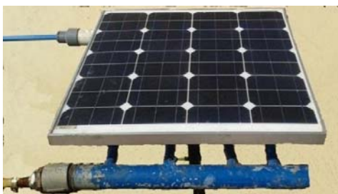
Fig 1 Photographic View of the PV Panel With cooling Arrangement
