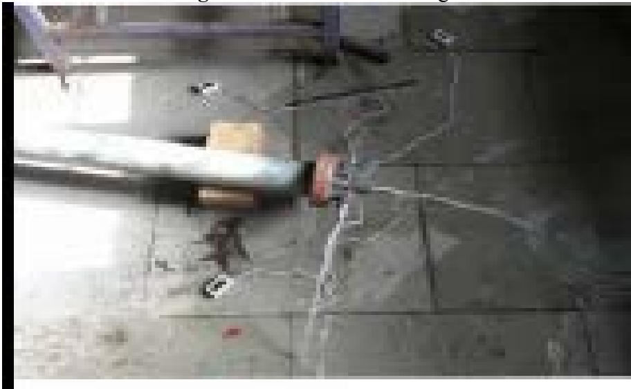
Figure 4 Outlet of heat exchanger
