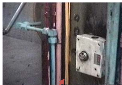
Liquid/ Lubrication Line
